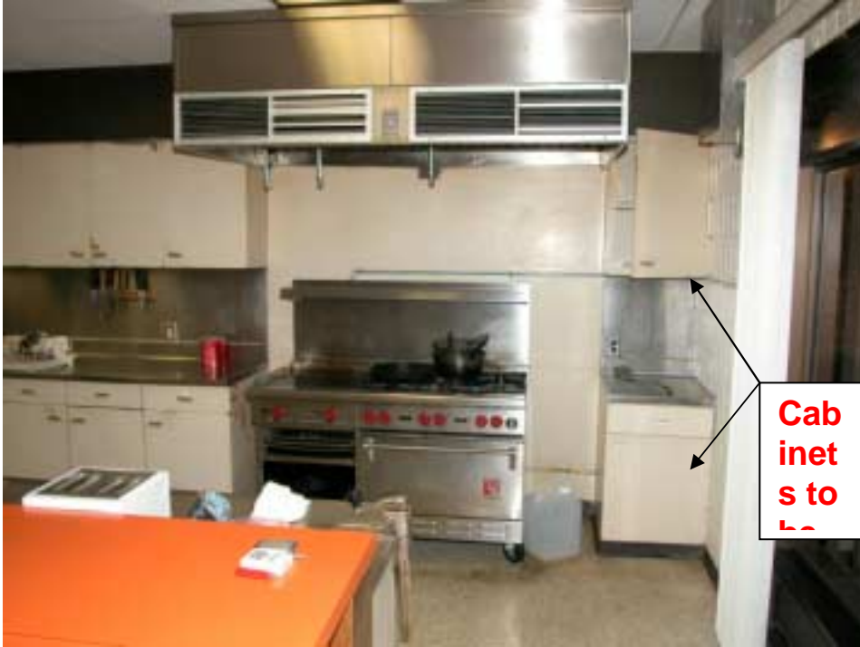
Figure 5 Station 4 The space behind the stove will be covered with stainless steel. The single base cabinet to the south of the stove should be changed from 21-1/2 inches to 36 inches. The hood range system will remain in place.
